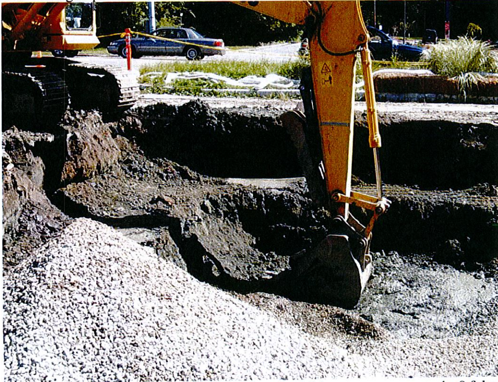
Limits of eastern wall of excavation with bench visible – tape on arm marks 8 ft bgs
