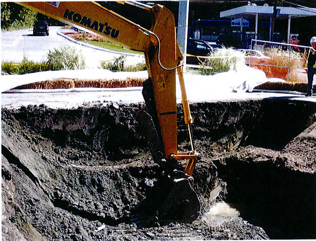
Bench along southern wall – excavator arm reaching depth of 8 ft bgs – GW at 8 ft
