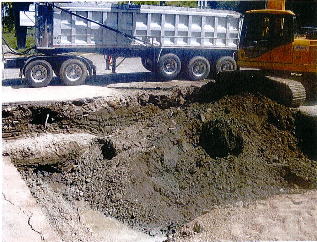
Direct loading impacted soil from excavation into trucks for transport to disposal facility
