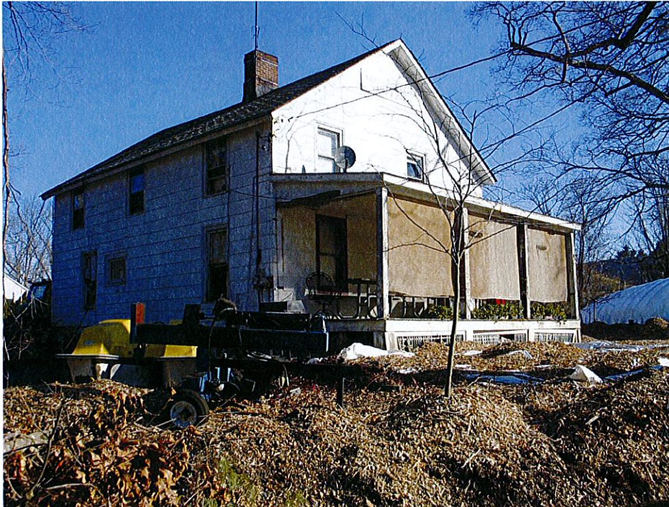
Photograph 6: Front (south) elevation of former dwelling on Zino's Nursery and Landscaping and Anthony's Power Equipment property, now retrofitted and used to repair lawn mowers. View looking northeast.
