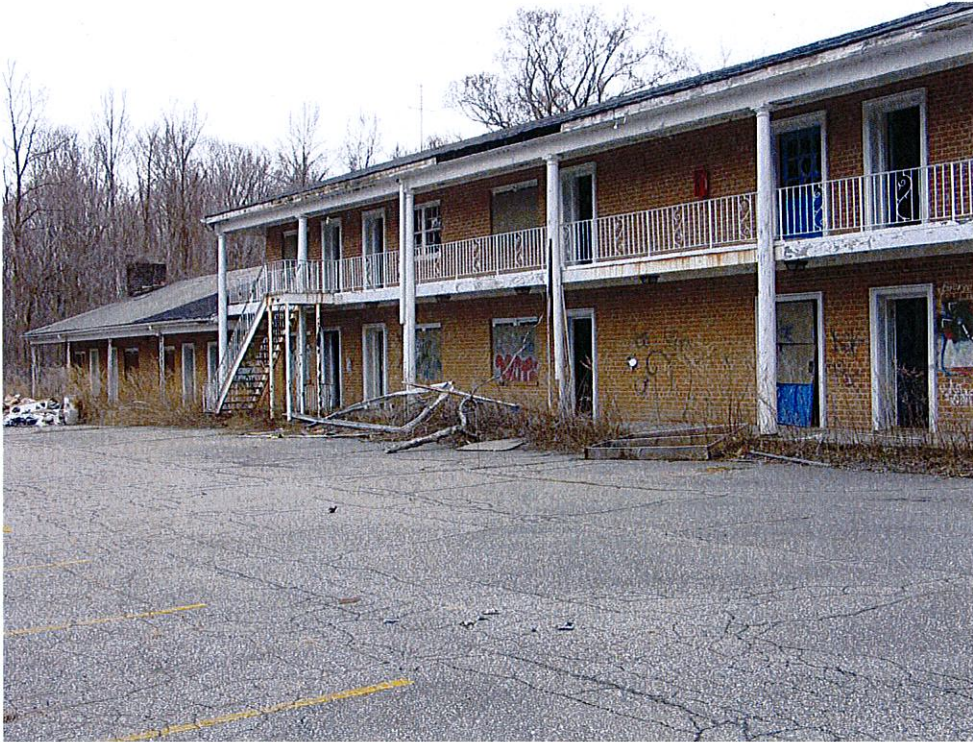
Photograph 21: Vacant motel showing western side of former motel building, where the rooms were located. View looking northeast.
