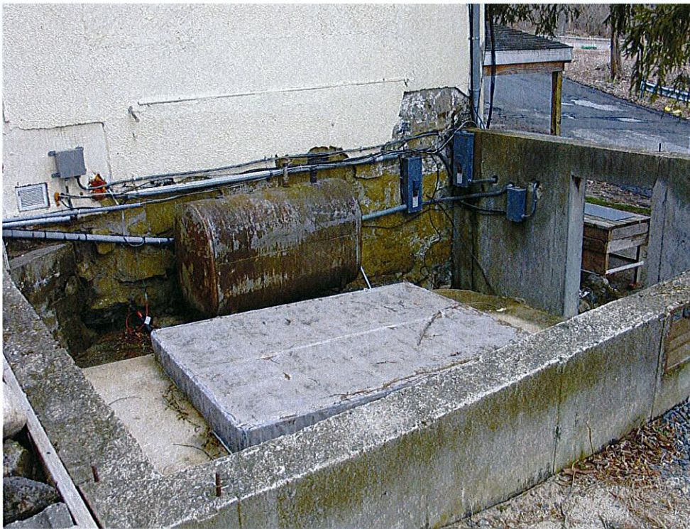
Photograph 2: Residence nearest Old Crompond Road showing exposed basement addition and stone walls under deteriorating stucco. View looking south.
