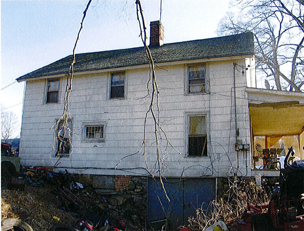
Photograph 11: Side (west) elevation of former dwelling on Zino's Nursery and Landscaping and Anthony's Power Equipment property, now retrofitted and used to repair lawn mowers, showing modified basement level. View looking east.
