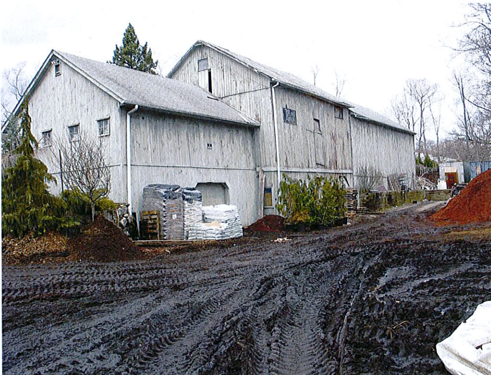
Photograph 14: Southeastern elevation of two story frame barn, comprised of three distinct sections. View looking northwest.
