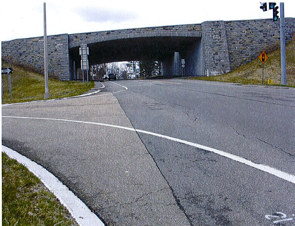
Photograph 42: Bridge carrying the Taconic State Parkway over Route 202/35, which was replaced in 2003-2006.
