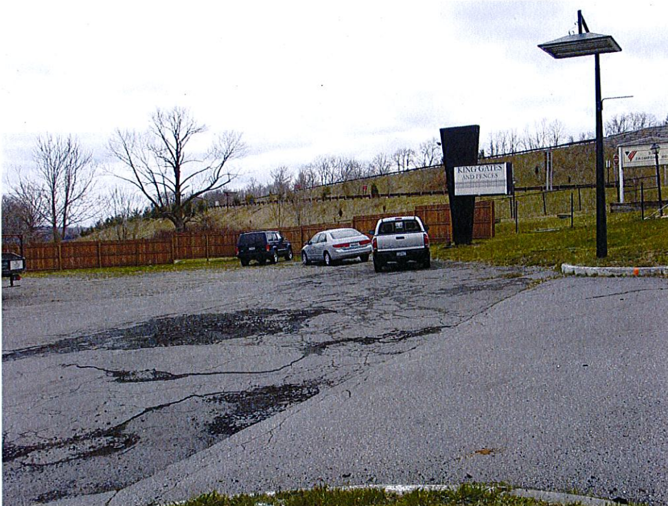
Photograph 35: Paved parking area associated with former gas station. View looking northeast, with Taconic State Parkway in background.
