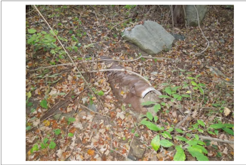
Rusted culvert with sediment found in North-Eastern corner of property
