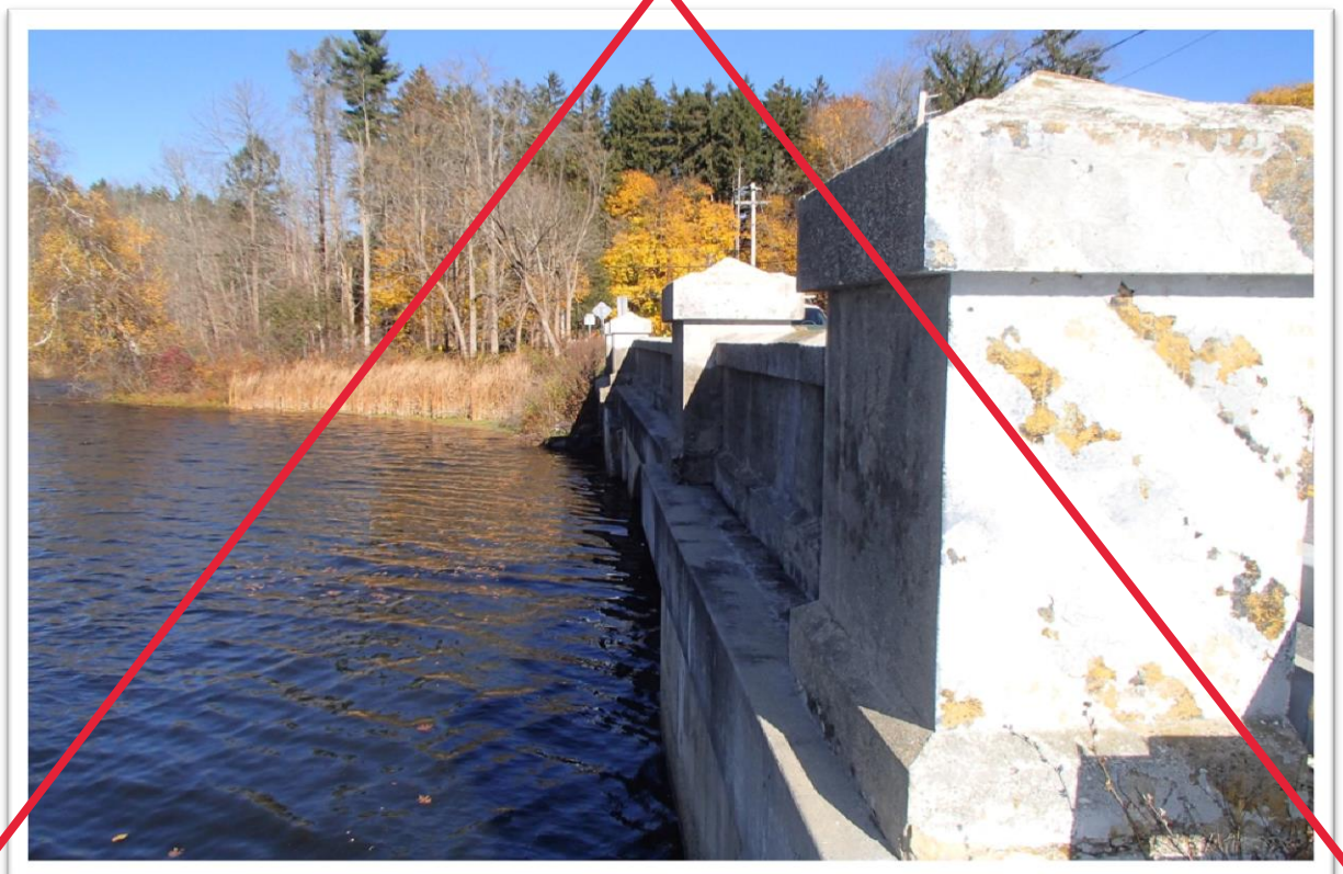
Photo H Cross River Inlet Bridge: View facing north from the southern side of the bridge showing existing bridge with wetlands in background across the water. Date Taken: November 7, 2018.
