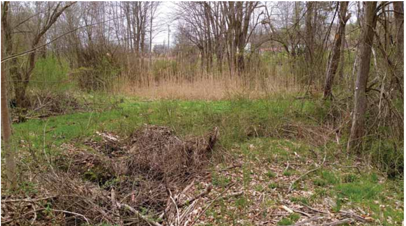
Wetland A with outlet from clogged culvert in foreground, Glen Rock Street in background
