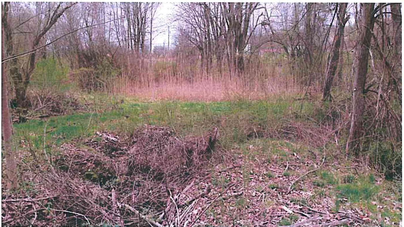
Wetland A with outlet from clogged culvert in foreground, Glen Rock Street in background
