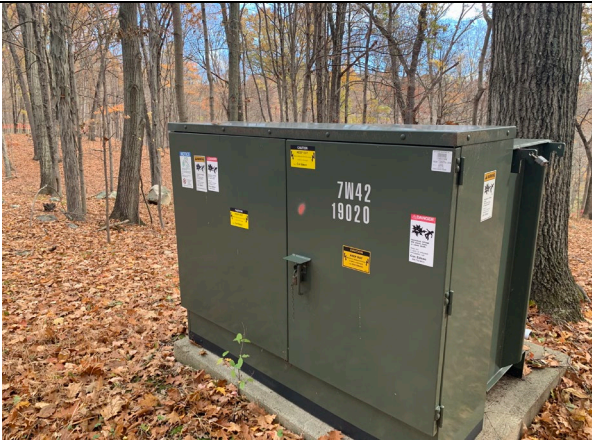
Photo 9: View of transformer in southern area of the Site.
