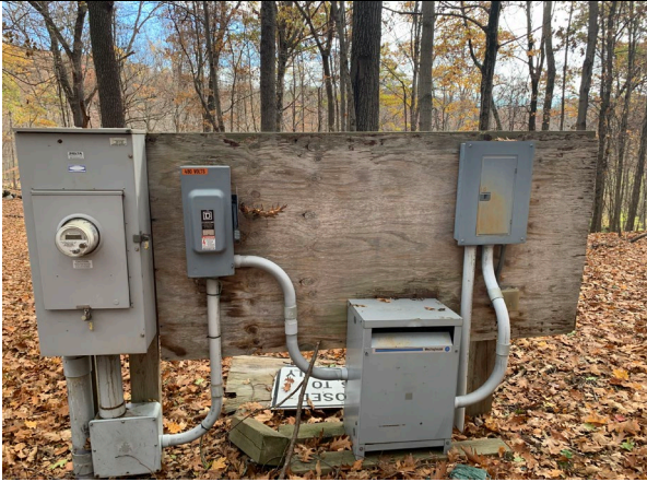
Photo 7: View of electrical utilities in the southern area of the Site.
