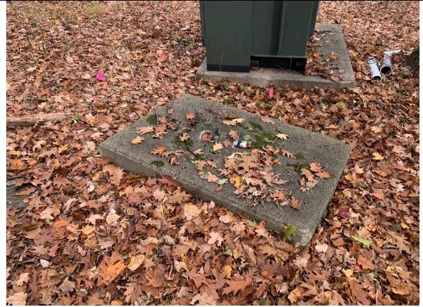
Photo 8: View of septic tank in the southern area of the Site.
