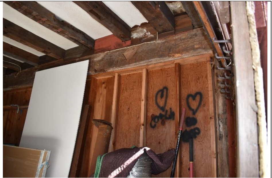
42. The interior of Building G has been substantially altered into the 21 st century, with the addition of a framed interior wall.
