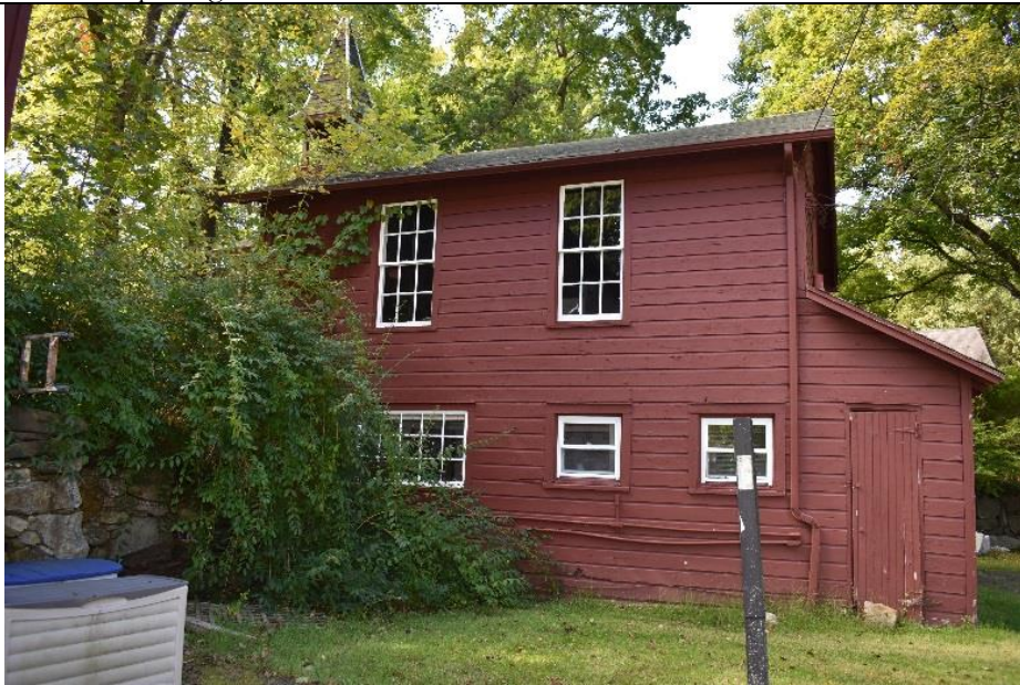
43: Building H is constructed adjacent to a stone retaining wall. View to the west.
