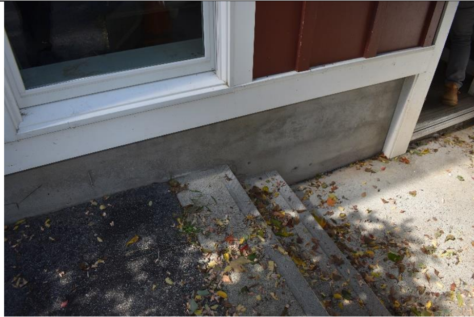
21. Building E features a modern concrete foundation on the southern and eastern walls.
