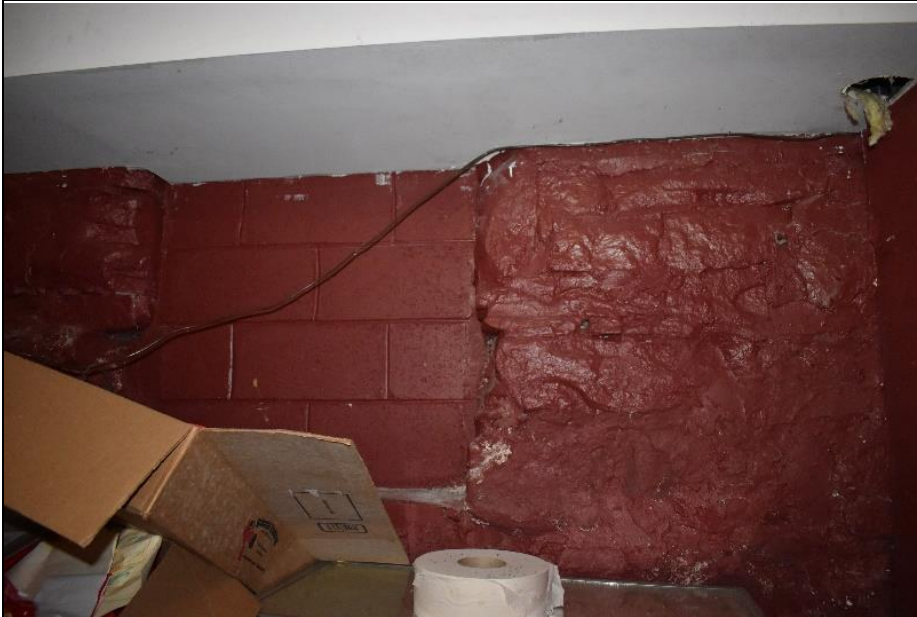
23. The original stall openings, from the original use as a barn, have been closed up with cinderblock. View of north wall of Building E.
