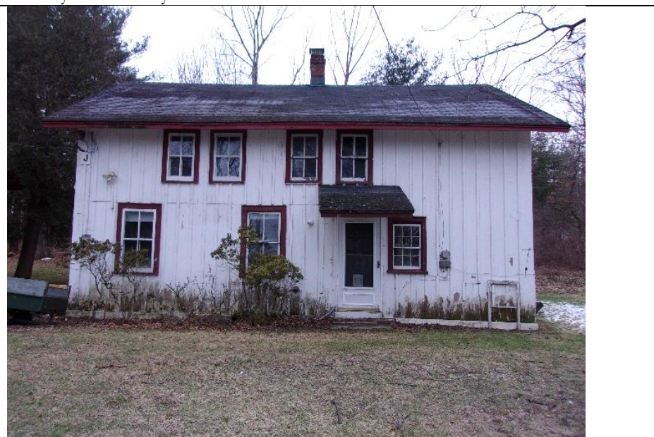
56 The fenestration on the exterior of Building J is uneven, and the windows are mixed in size, and pattern.
