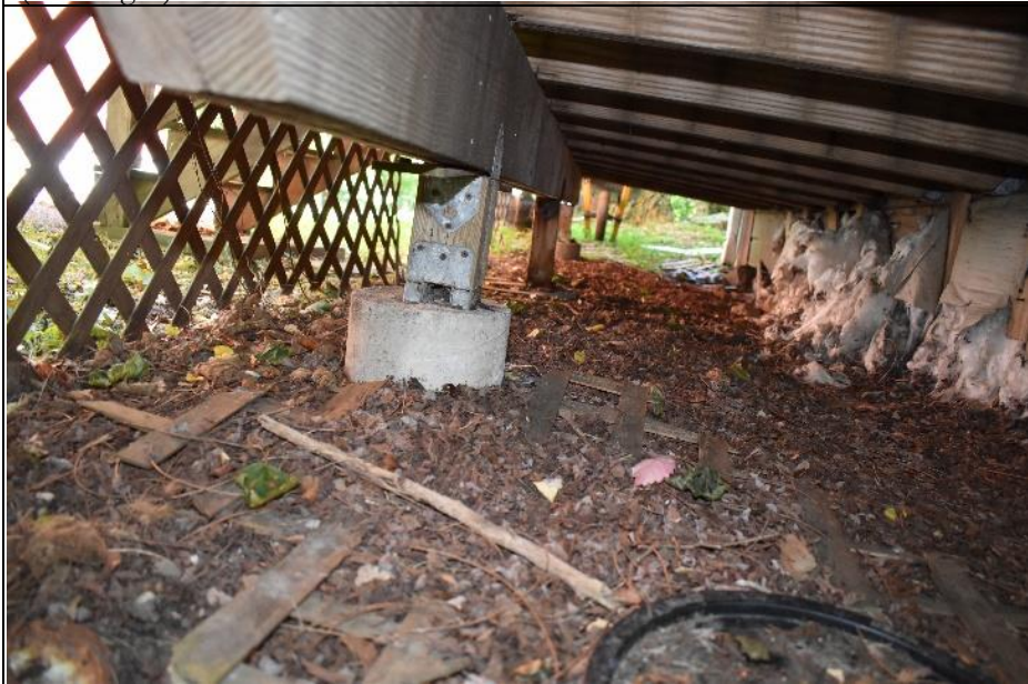
31. The footings and support systems for the additions of Building E all date to the mid to late 20 th century.
