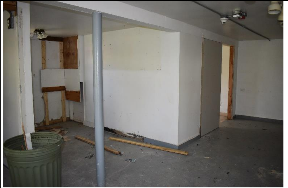
46. The interior of the basement of Building H features a concrete floor, metal (steel) lally columns and other 20 th century materials.
