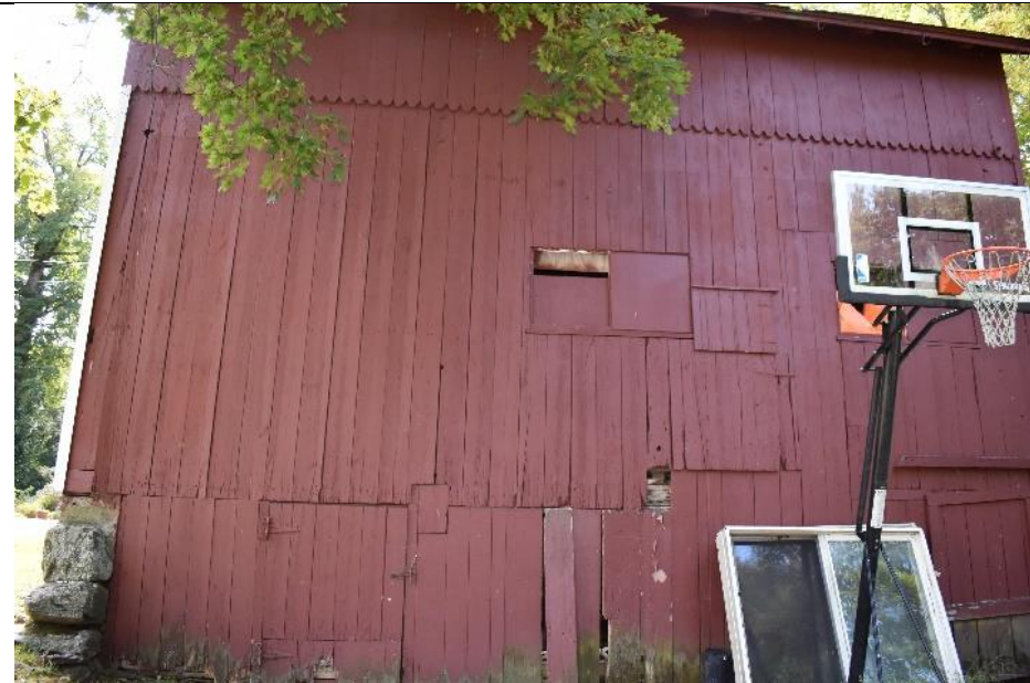
35. Multiple openings and access points are visible on the northern elevation of Building G.
