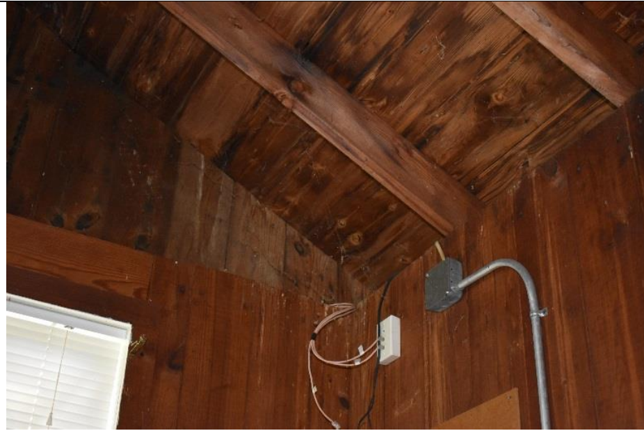
45. The interior features platform framing and 20 th century construction materials Building H.
