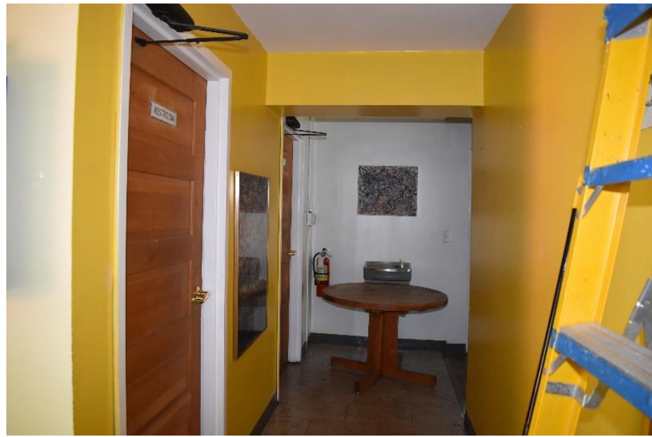
25. The interior of Building E has been substantially renovated in the 20 th and 21 st Century.
