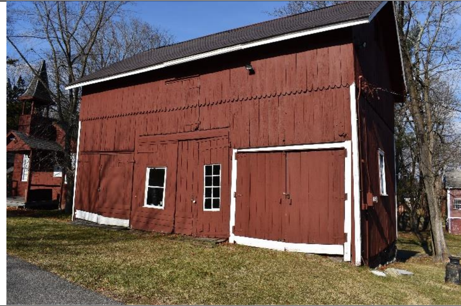
33. View northwest of Building G, the entrances and openings have been modified over time.
