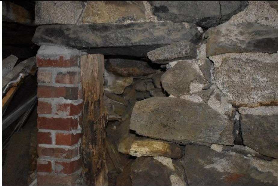
37. The foundation of Building G is a mix of timber, brick and stone.
