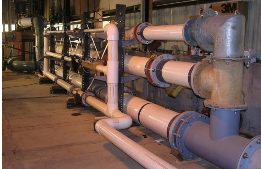
Figure 5 Photograph Showing Laboratory Flow Meters
