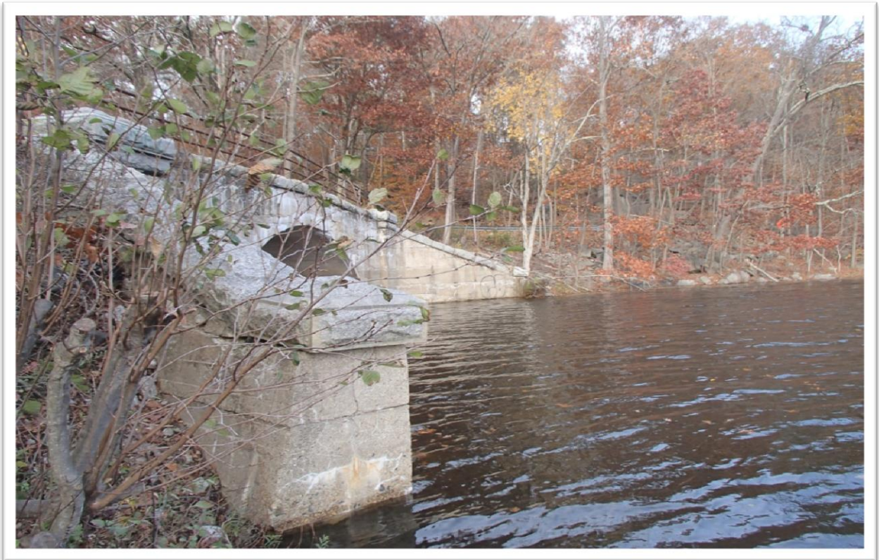
Photo B Baptist Church Road Bridge: View facing east from the western side of the bridge showing existing bridge and New Croton Reservoir. Date Taken: November 7, 2018.
