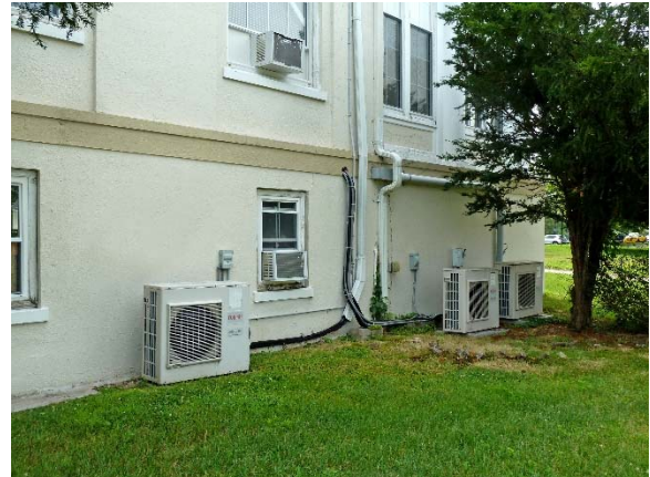
In-window air conditioning units; multiple split system condensing units with conduit overlapped by downspout
