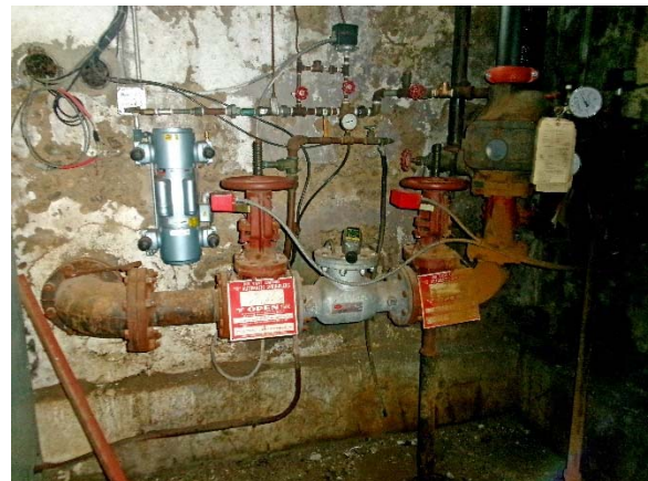
Basement mechanical room: controls for sprinkler system
