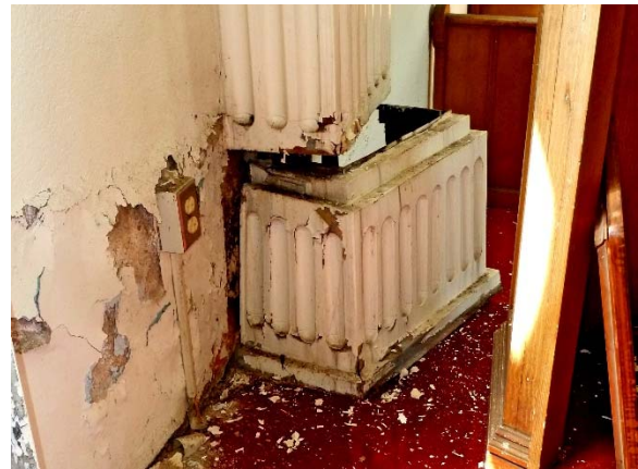
Chapel, south wall by sanctuary: sheet metal pilaster/tie cover disconnected; peeling paint on exterior wall and cover
