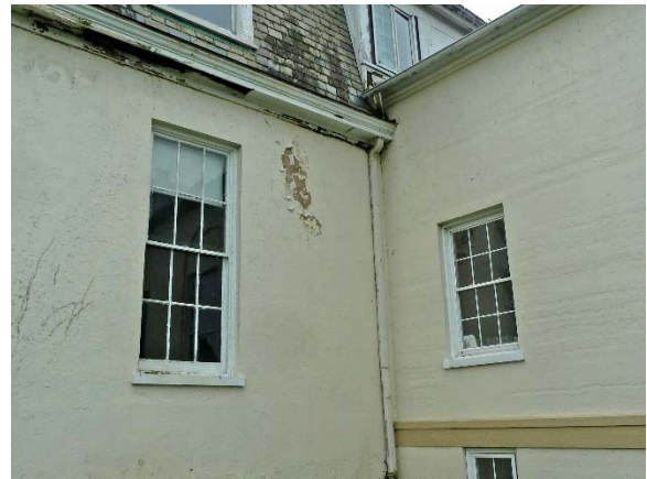
Chapel, north elevation: roof soffit very deteriorated and open; peeling paint on wall; downspout at corner with pavilion
