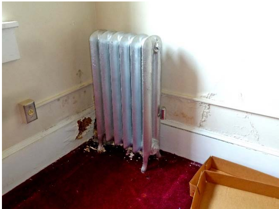
Peeling & bubbling wall and baseboard finishes around steam radiator suggests ineffective or failing controls
