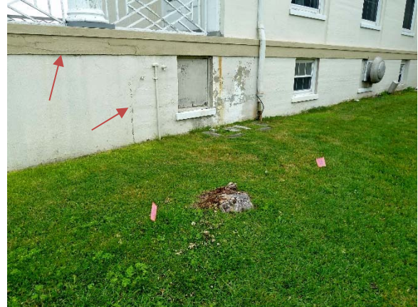
East Pavilion, west wall: cracks at basement level where interior spaces begin & at water table/edge; peeling paint
