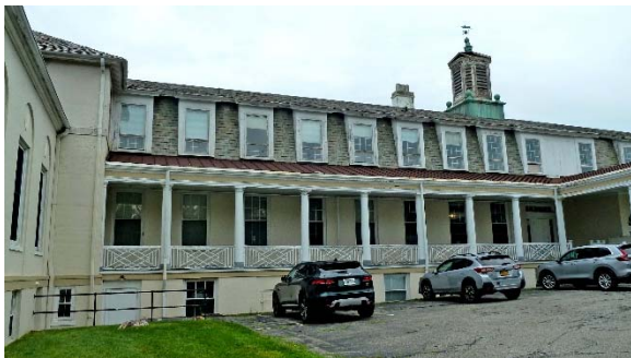
Central Addition (1897): porch in fair condition with likely original standing seam roof, replacement balusters, parking
