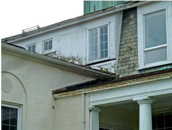
Dormer above East Pavilion: wood panels adjacent to roof very deteriorated from splash back; disconnected triangular panel
