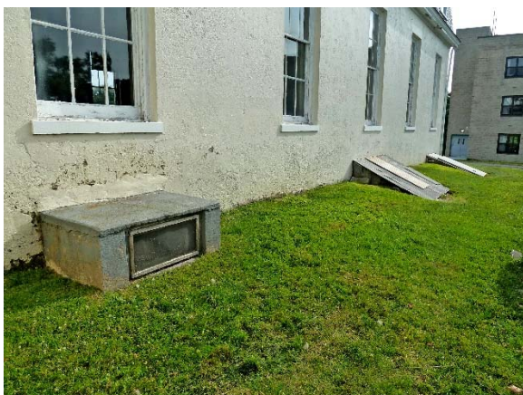
Chapel, south elevation: peeling paint and repairs at lower walls; access point to basement level
