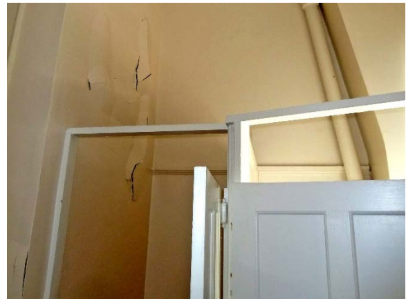
Bathroom at western end of hall: painted finishes bubbling, settling, and falling off at partition wall to linen closet
