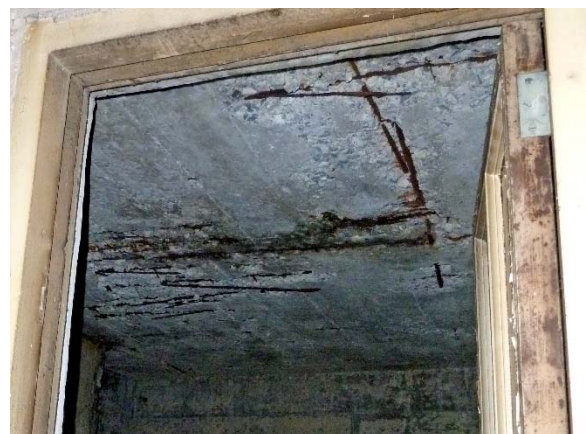
Underside of West first floor entry portico: concrete slab with multiple rebar visible & rusty near the deteriorated surface
