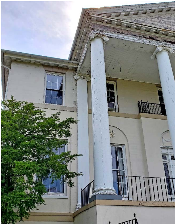
Details of portico: flaking paint on wood pediment, columns, & concrete wall; severely deteriorated volutes on Ionic capitals
