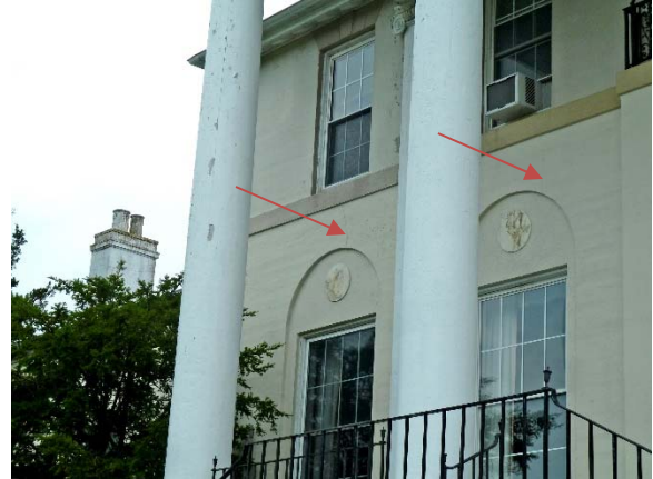
Vertical cracks in concrete wall between first & second floor window openings (all bays of portico)
