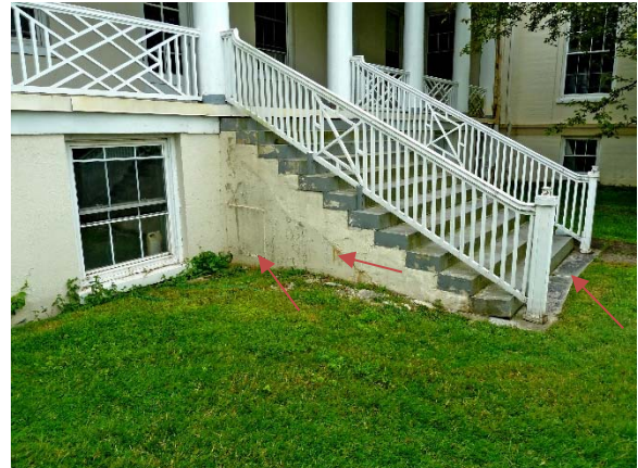
North porch stairs: visible structural cracks on side wall(s); displaced & rotated lowest two stairs/treads; peeling paint
