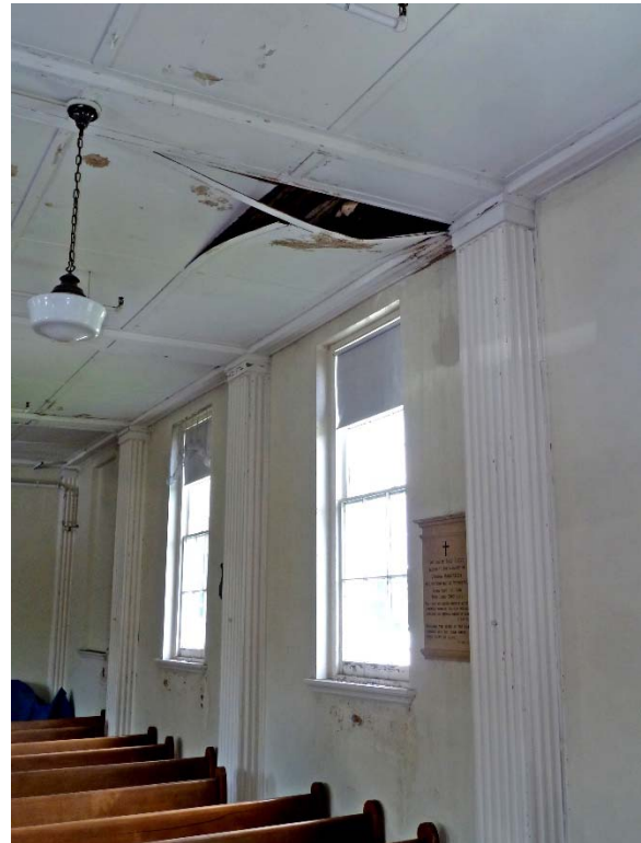
Chapel, north windows: disconnected fiber board applied atop beadboard; deteriorated finishes below window sills
