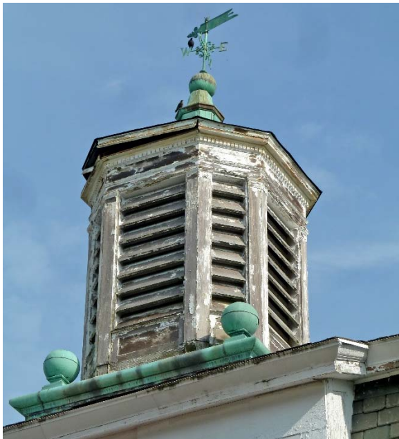
View of existing louvered cupola from southeast: portion of roof lifting upward; little paint remains; copper details; birds
