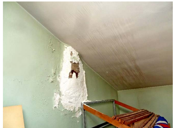
Records room at East Pavilion stair landing: very deteriorated plaster with repair attempt; water-stained ceiling
