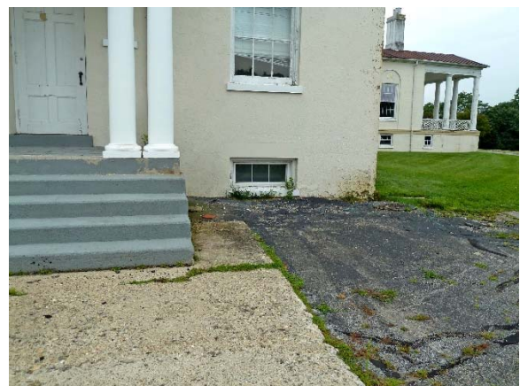
Chapel, east elevation: peeling paint along northeast corner of building & concrete stair; macadam driveway with repairs
