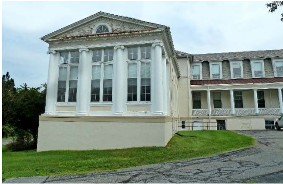
South Pavilion (enclosed), 1924 addition: peeling paint & rusting at pediment & engaged Ionic columns
