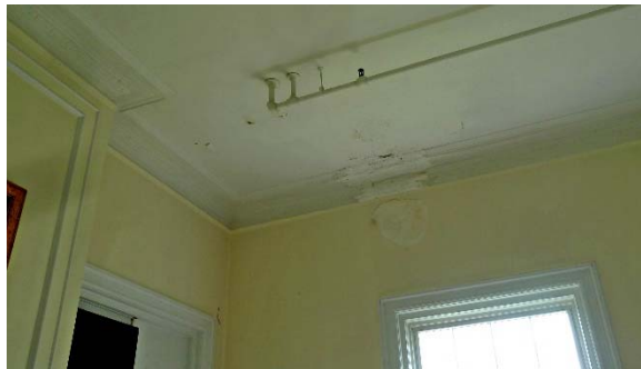
East Pavilion (1924); deteriorated plaster cornice with repair, likely due to water infiltration from roof/gutter; sprinkler pipes
