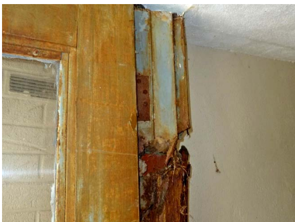
Exterior basement door, at West Elevation: steel frame severely rusted & disconnected with bird nest inside
