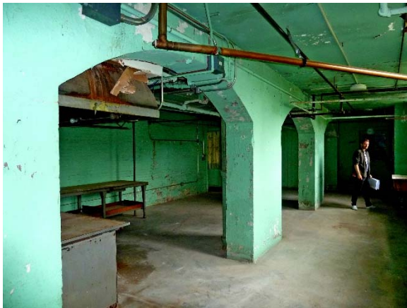
Structural arches in historic laundry (north rooms) providing structural support to exterior walls above; peeling paint
