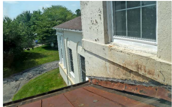
East wall of 1924 Addition: peeling paint and visible staining on concrete walls; original porch roof and flashing with repairs
