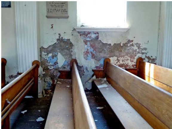
Chapel, south wall: severely deteriorated finishes below window sills, allowing view of previous paint layers & bare concrete
