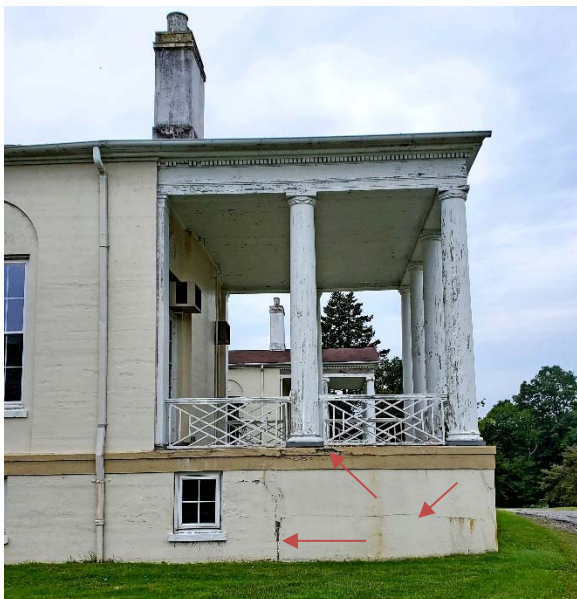
East façade of East Pavilion: horizontal & vertical cracks at basement level; broken edge of porch floor; Tuscan columns
