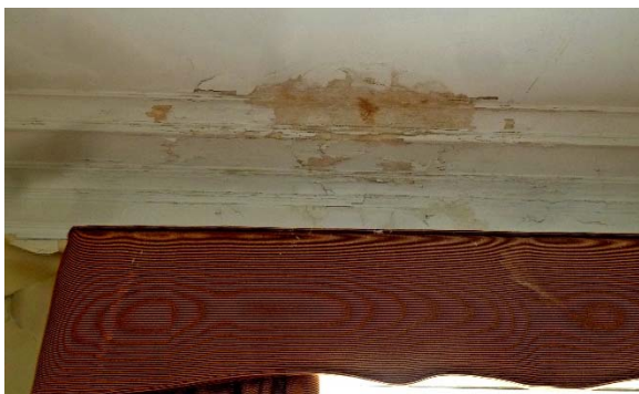
West Addition (1924), north parlor: deteriorated plaster cornice above window valance (similar condition, south parlor)
